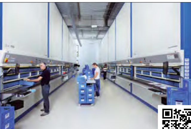
Small parts are picked quickly and efficiently from 12 Hänel Rotomat® storage carousels
